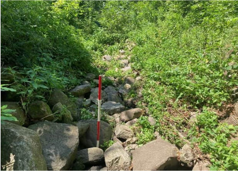
Photo 2 Channel looking downstream. Becoming overgrown
