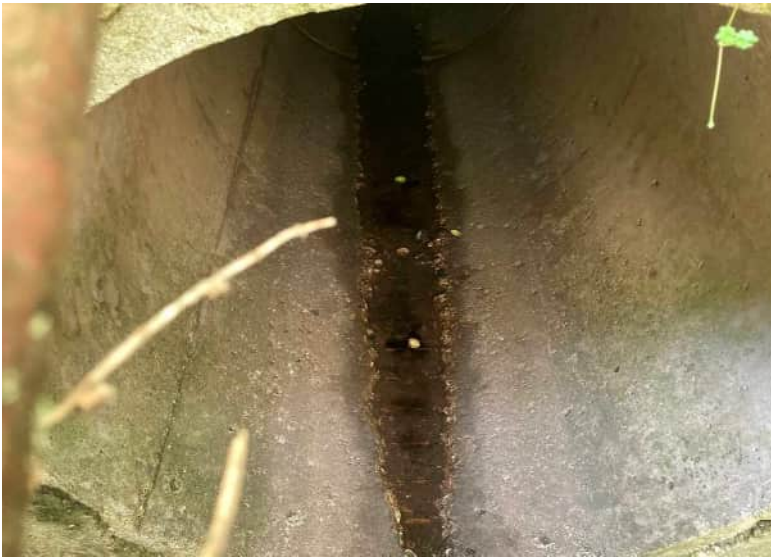
Photo 10a 48" RCP outfall Missing concrete in invert
