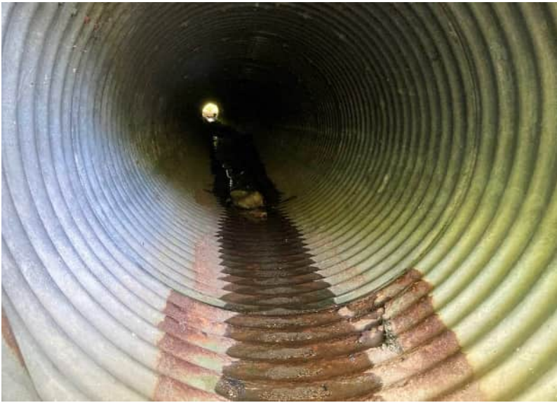
Photo 14b Middle outfall - 36" CMP Bend along length
