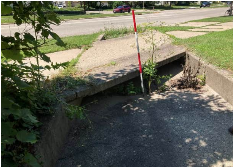
Photo 6 Raised sidewalk exposed rebar on left side 6' w x 12" h at edge, 13" h at midpoint
