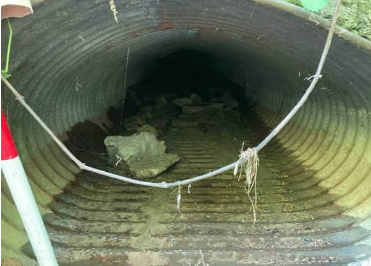
Photo 16a ~43" x ~26" CMPA (42" x 29" = likely standard size) Rocks and sediment build-up within culvert
