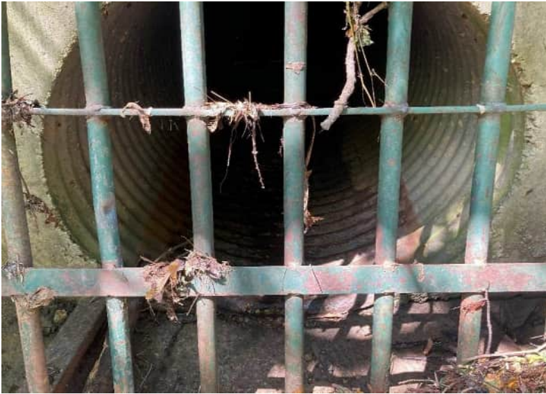
Photo 11a Some Corrosion on Left channel outlet
