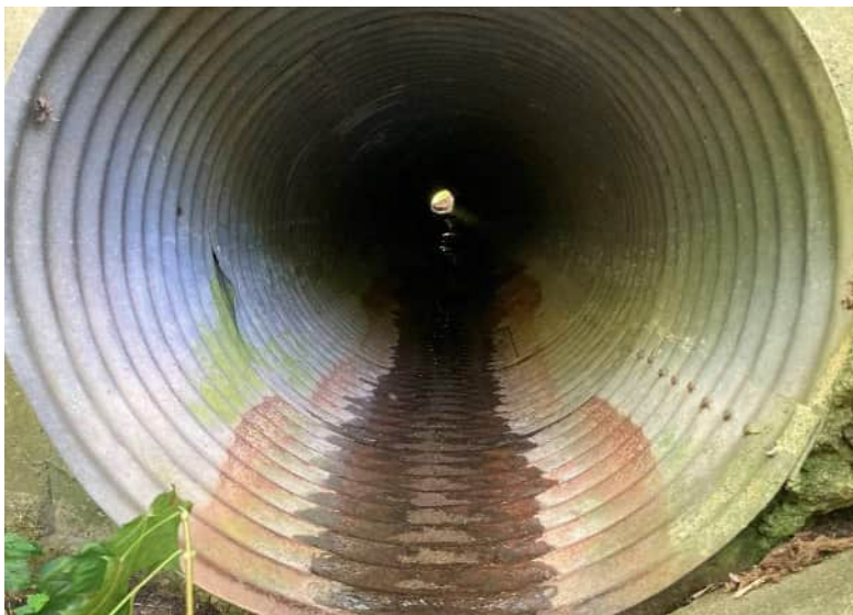
Photo 14a Left outfall - 36" CMP Downward bend along length
