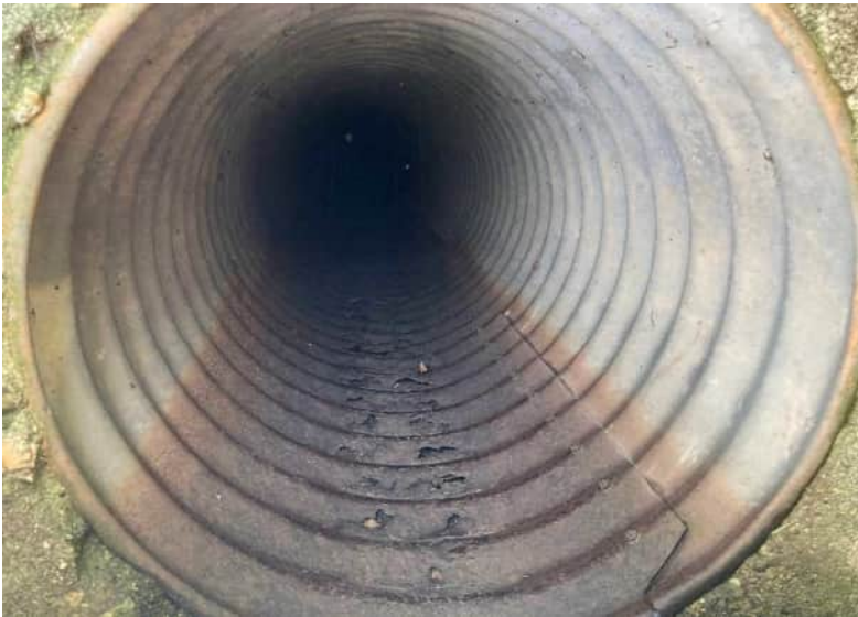
Photo 3a 18" CMP Corrosion on bottom
